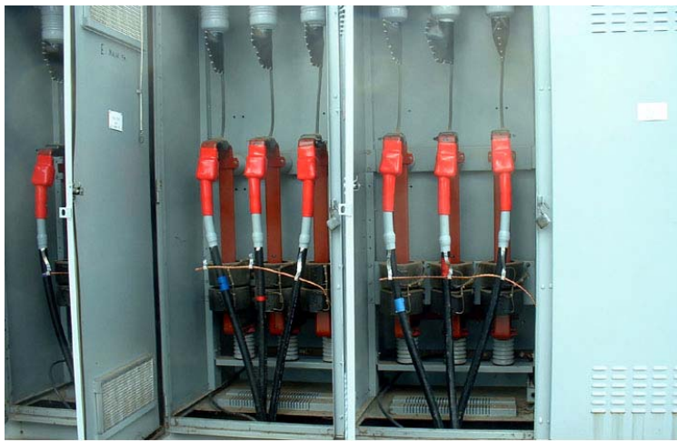
Underground 15,000 feeder cables in rear of metal clad switchgear
