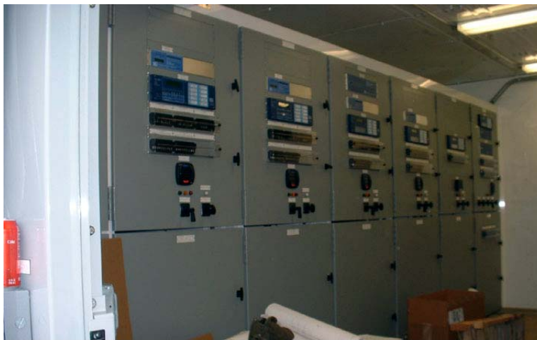
Relays and switches on panels and switchgear, if bumped can lead to large scale power outages
