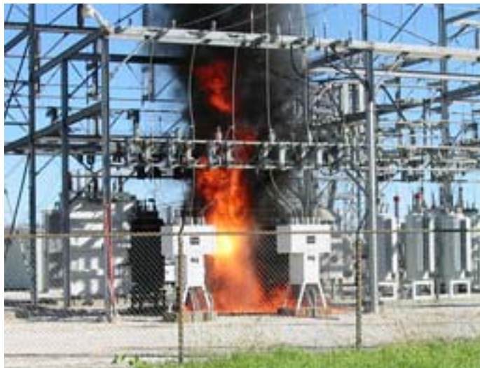
Transformer Oil Fire on an overheated 69,000 volt substation transformer
