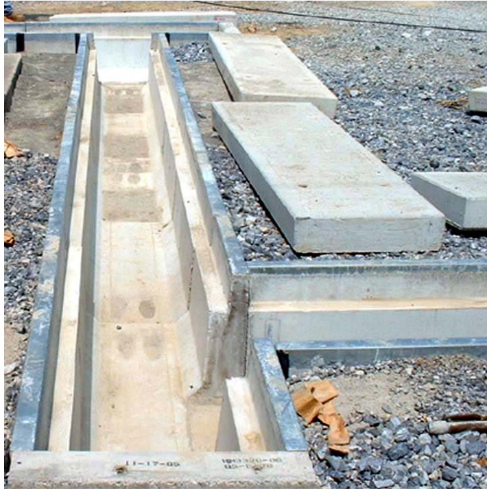
Traffic rated precast cable trench with lids removed
